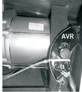
Figure B - Review the location of the AVR (Automatic Voltage Regulator). This item may eventually need to be replaced when they wear out.
